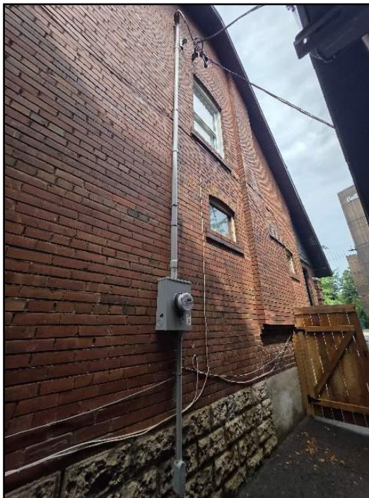
15. Overhead - cable type not determined
