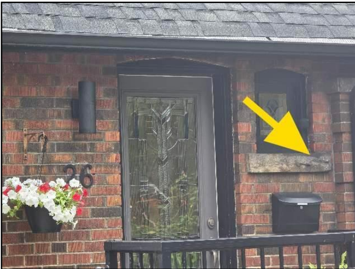
11. Paint and Caulking - deteriorated / miss
