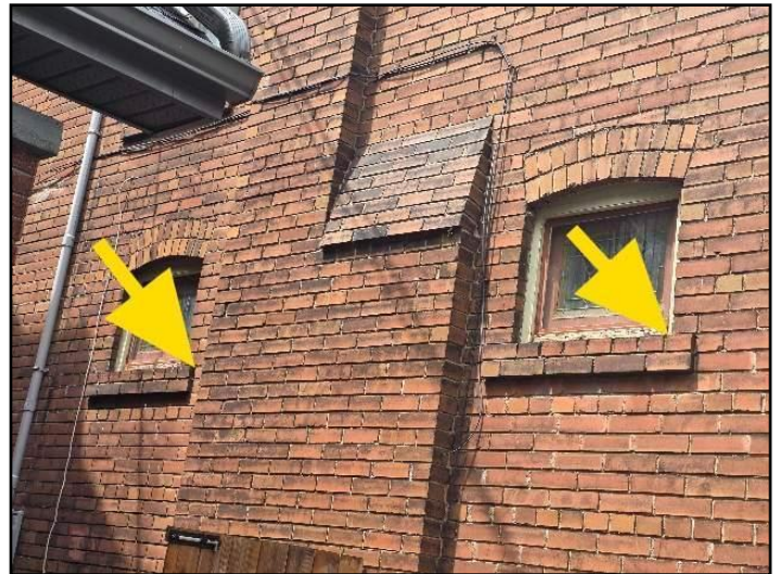
12. Paint and Caulking - deteriorated / miss
