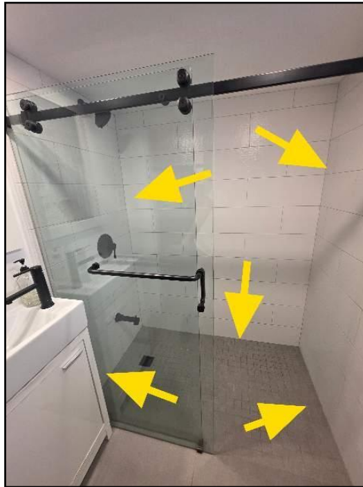
40. Caulking loose, missing or deteriorated
