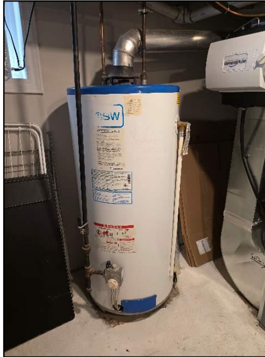
39. High failure probability
