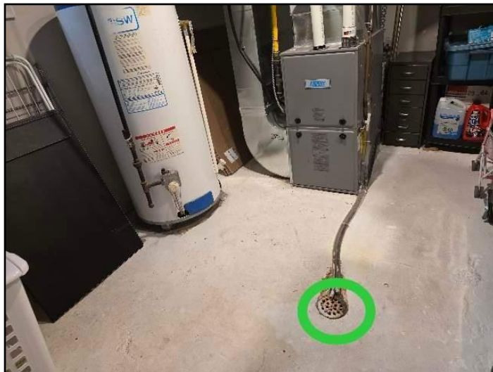
37. Near heating system
